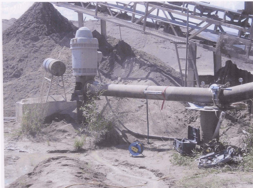
New Crusher Well (old well at right below valve)
