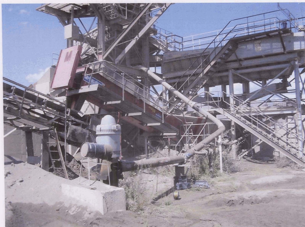
New Crusher Well, pipeline, and one of the gravel washing facilities
