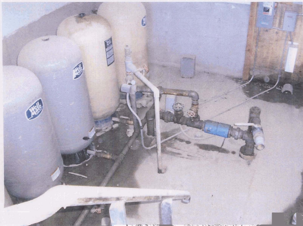
Shop Well showing discharge line and pressure tanks
