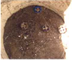
SHUT OFF VALVES FOR EACH DOMESTIC AND M...
