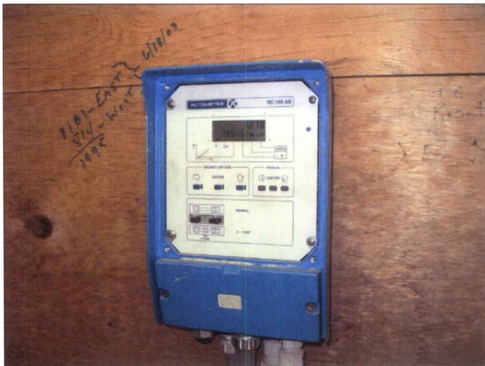
Photo 6: Digital display for mag meter located inside pit booster pump house.
