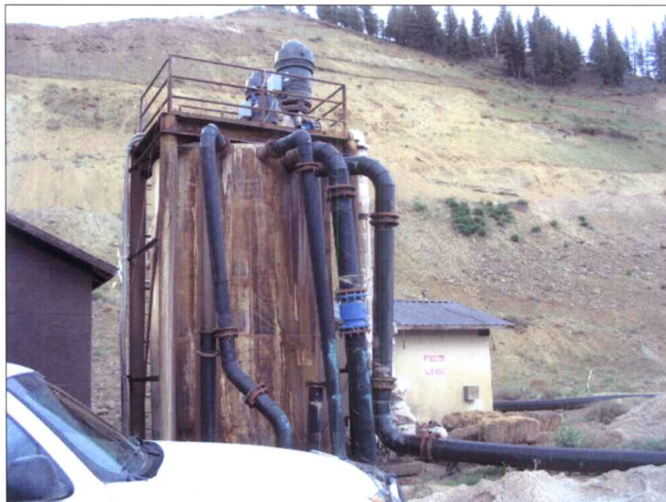
Photo 4: Upper pit booster station with two 300-hp vertical turbines receives water from pit and discharges to fresh water or reclaim water head tanks and/or tailings pond, and then to the mill.
