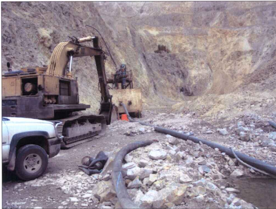
Photo 3: Pumping station at intermediate level pit lifts water to upper pit booster station.
