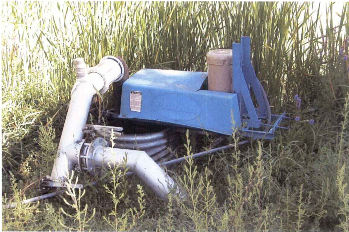
- POD. Line splitting to the right supplies water to POU in WR# 63-12113. Line going straight serves neighboring WR# 63-276C.
