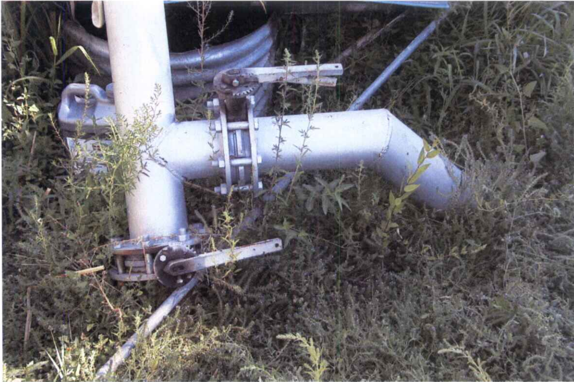
- Lockable control devices.
