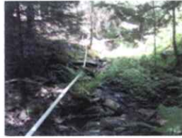
HYDRO POWER PIPE
