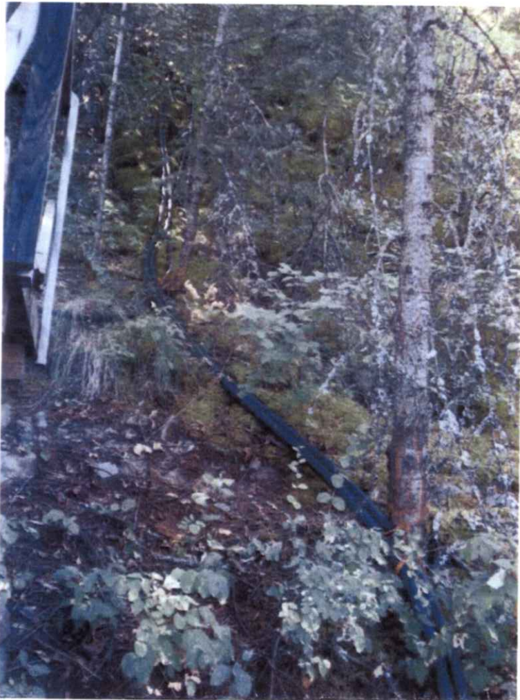
95-8817 water & Elect. line to lake pump
