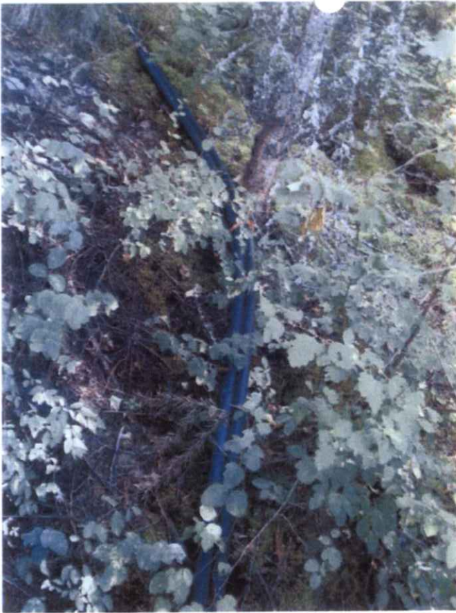
95-8817 Water and Electrical Line to pump.
