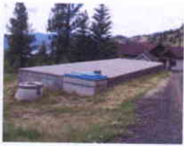
30,000 GAL HOLDING TANK
