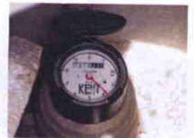
METER FOR WELL #2
