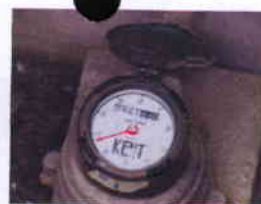
METER FOR WELL #1
