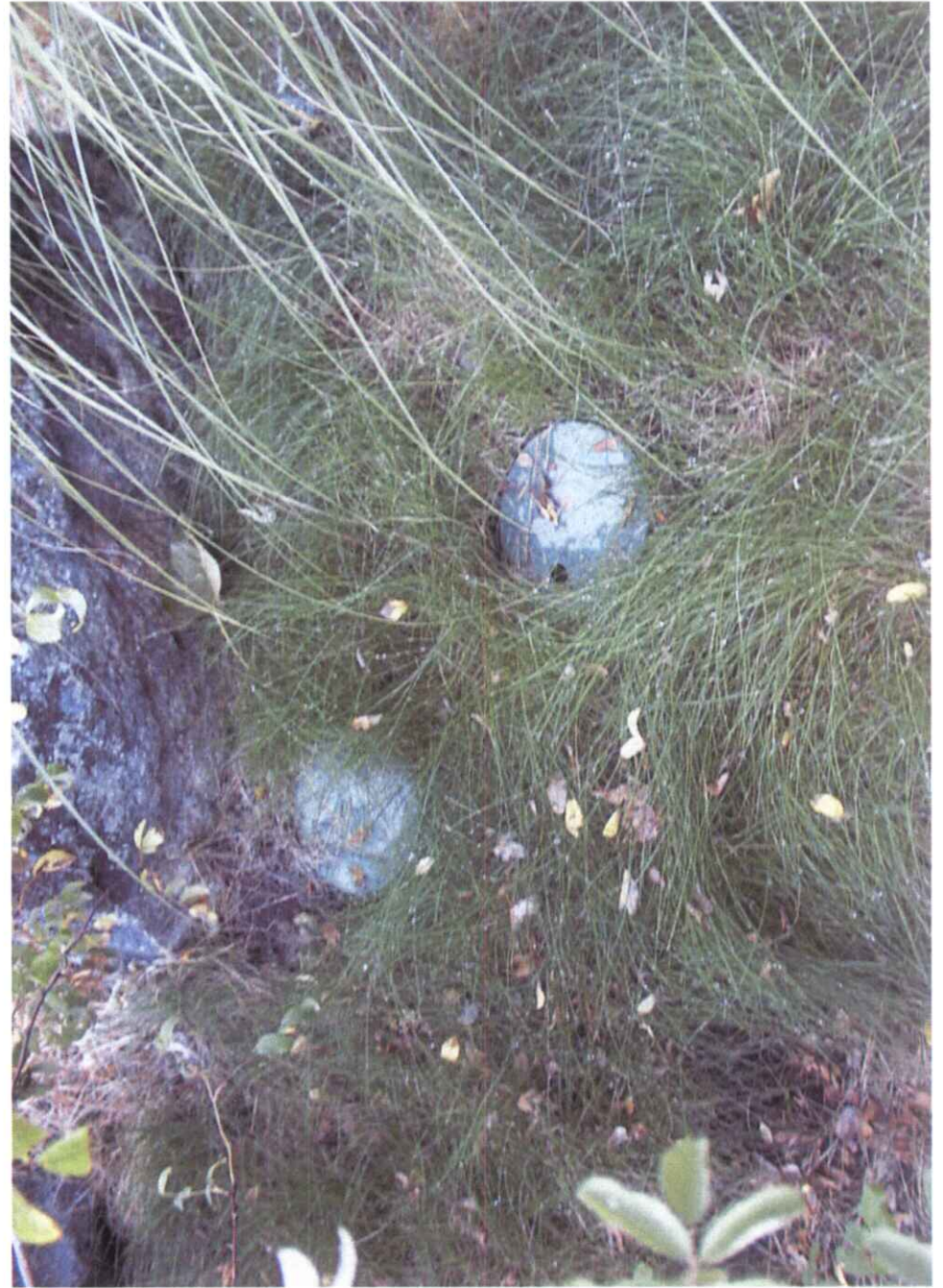
VALVE BOXES LOCATED IN GRASS BEHIND EACH WATERFALL.
