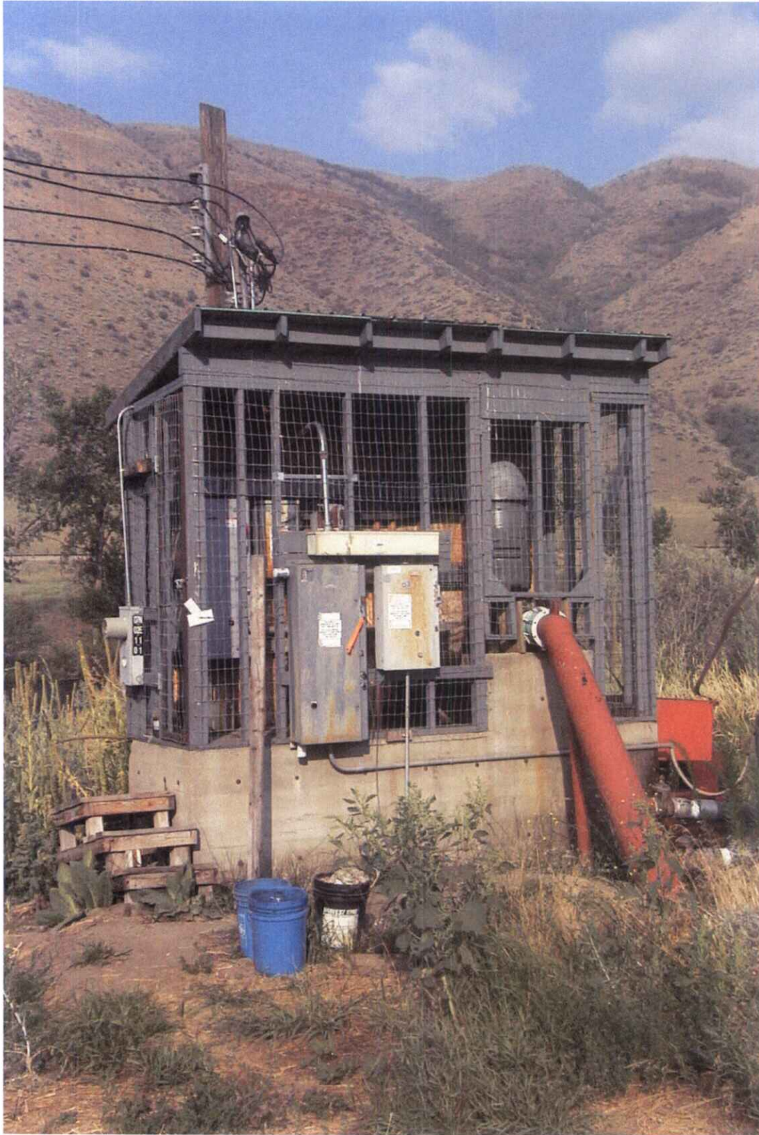
- Main pump house, 100hp pump inside.
