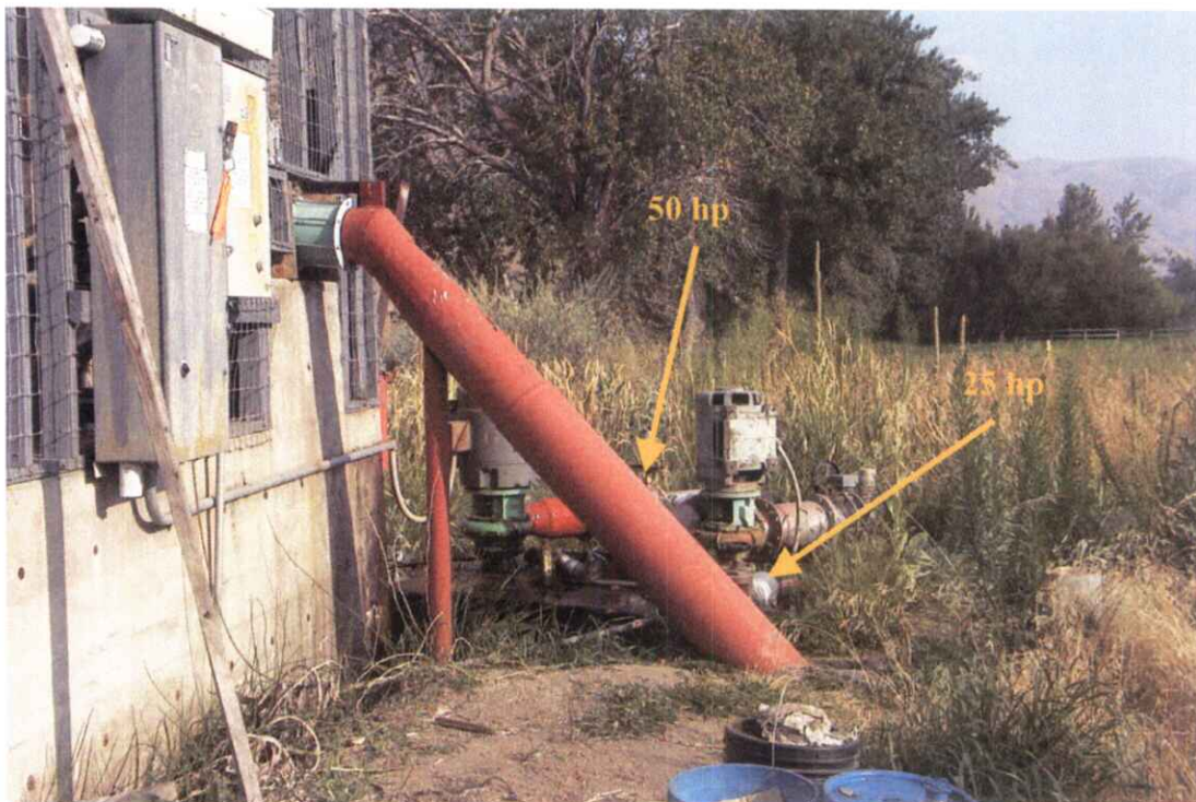
- 50 (left) and 25 (right) hp pumps that provide supplemental pressure when needed. Yellow arrows indicate where water enters mainline from these pumps.
