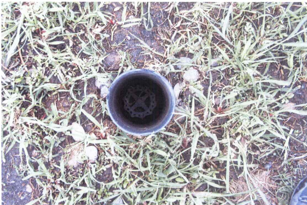
- Mainline T diverting water to owner's property
