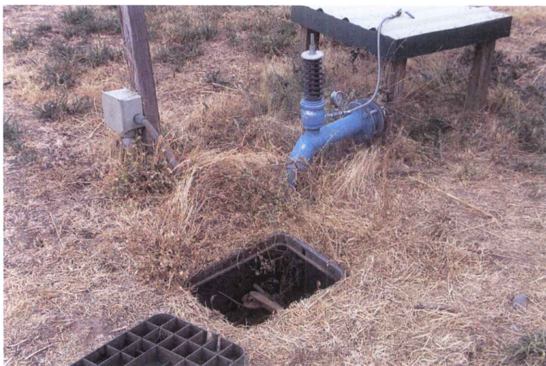
- Lockable control device. Blue pipe directly above is inlet into system from overlapping right 65-3803C. Source (pond) of 65-3803C is immediately to the right from where picture is taken.
