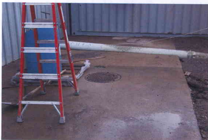
Top of 10,000 Gallon reservoir at Batch Plant
