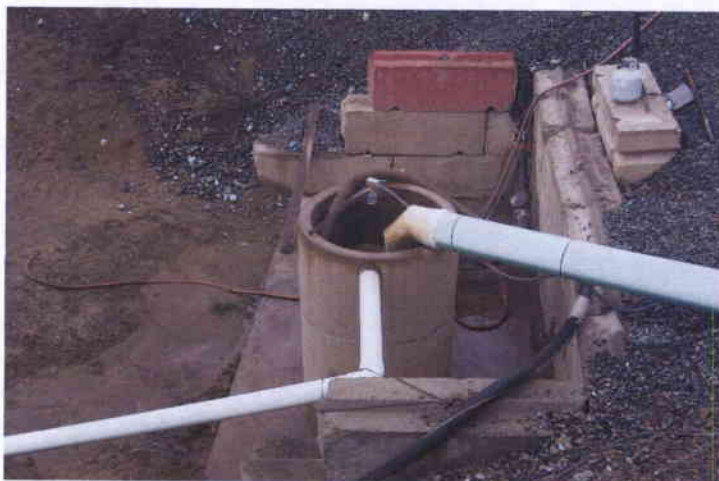
wastewater line carrying sediment from wash plant to pump & line leading to settling pond #2
