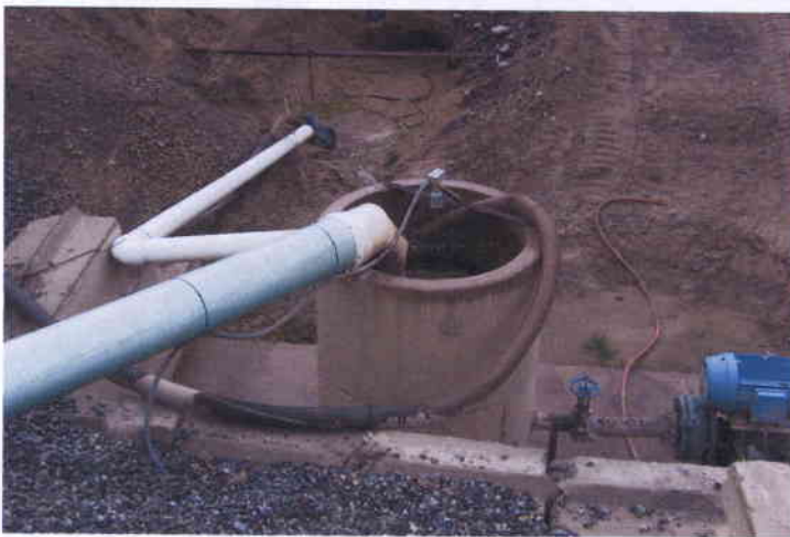
wastewater line carrying sediment from wash plant to pump & line leading to settling pond #1
