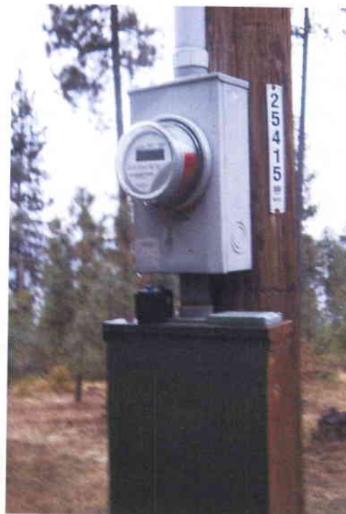
Electrical Meter for Pump in submersible cage
