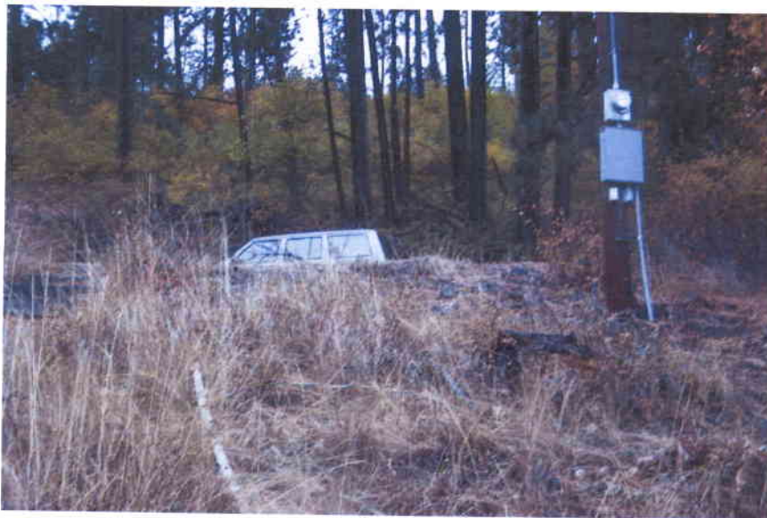
Electrical meter for submersible pump & water line leading under Sublimity Trail road toward home
