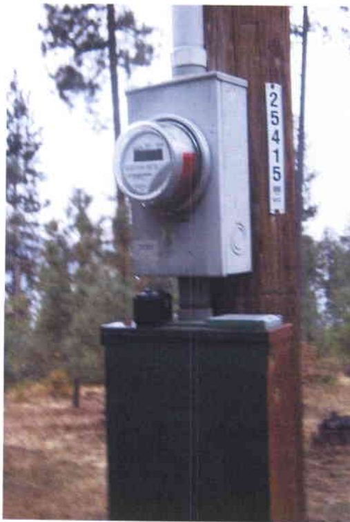
Residence & domestic pump water electrical meter
