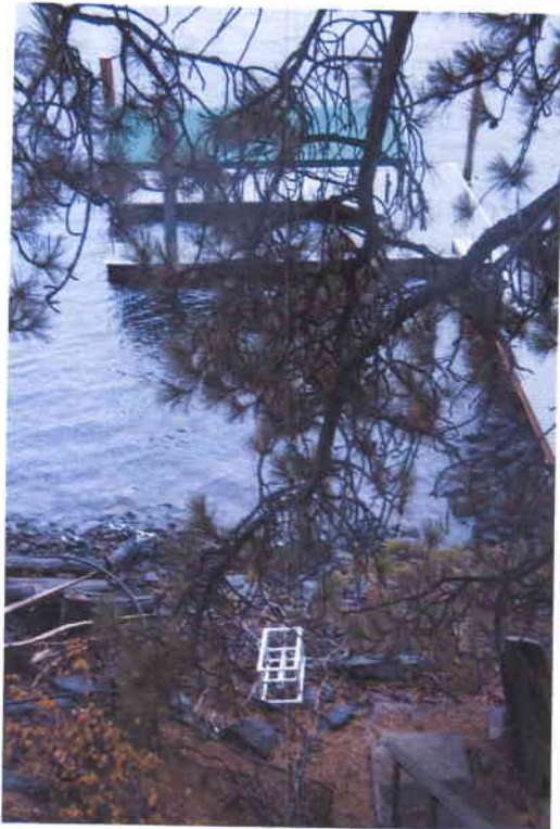
Submersible pump cage on shoreline next to dock Point of Diversion (POD)
