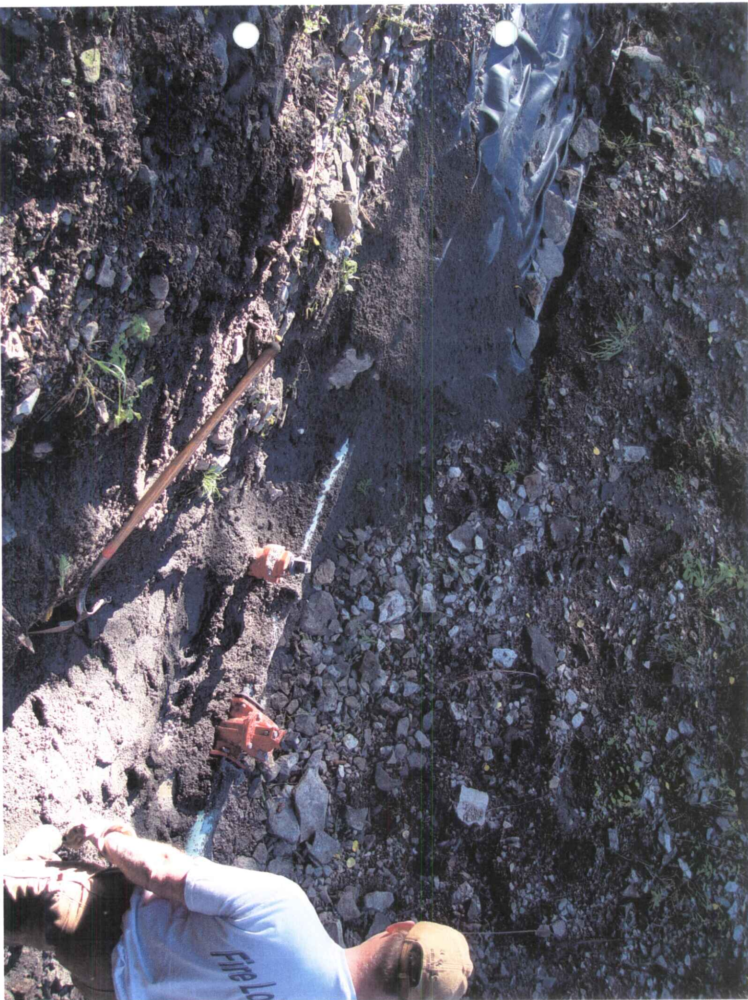
Membrane over washed Rock. Pipe exiting collection area & valve gates
