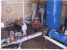
SYSTEM 1 AND WELL #1.JPG
