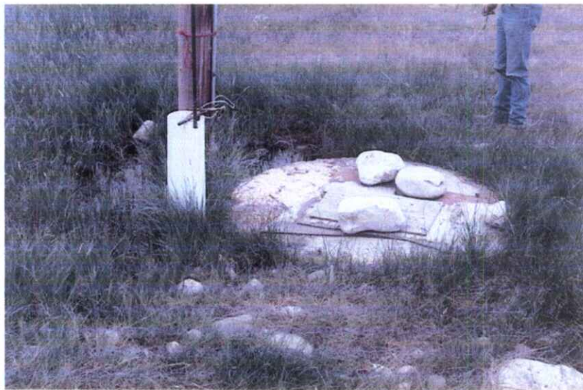
74-7387 Buried 6 foot by 8 foot cistern with 1 hp pump. 07/24/07
