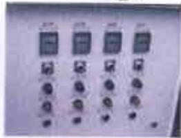
PUMP CONTROL PANEL
