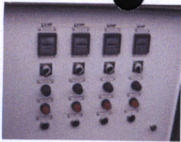
PUMP CONTROL PANEL
