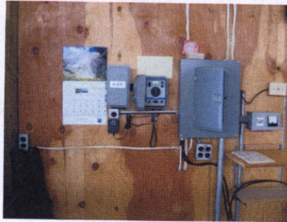
92-7223 Irrigation Zone Electrical Controls In Garage
