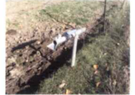
STAND PIPES FOR IRRIGATION
