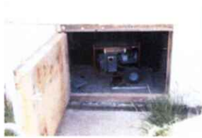
92-10008 Generator to power water system
