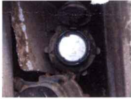
METER FOR WELL #2.jpg
