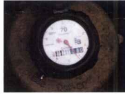
METER FOR WELL #3.jpg
