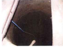
PIPE FROM STREAM AND PIPE TO HOUSEWITH P...
