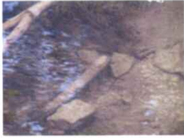
INLET PIPE FOR PUMP
