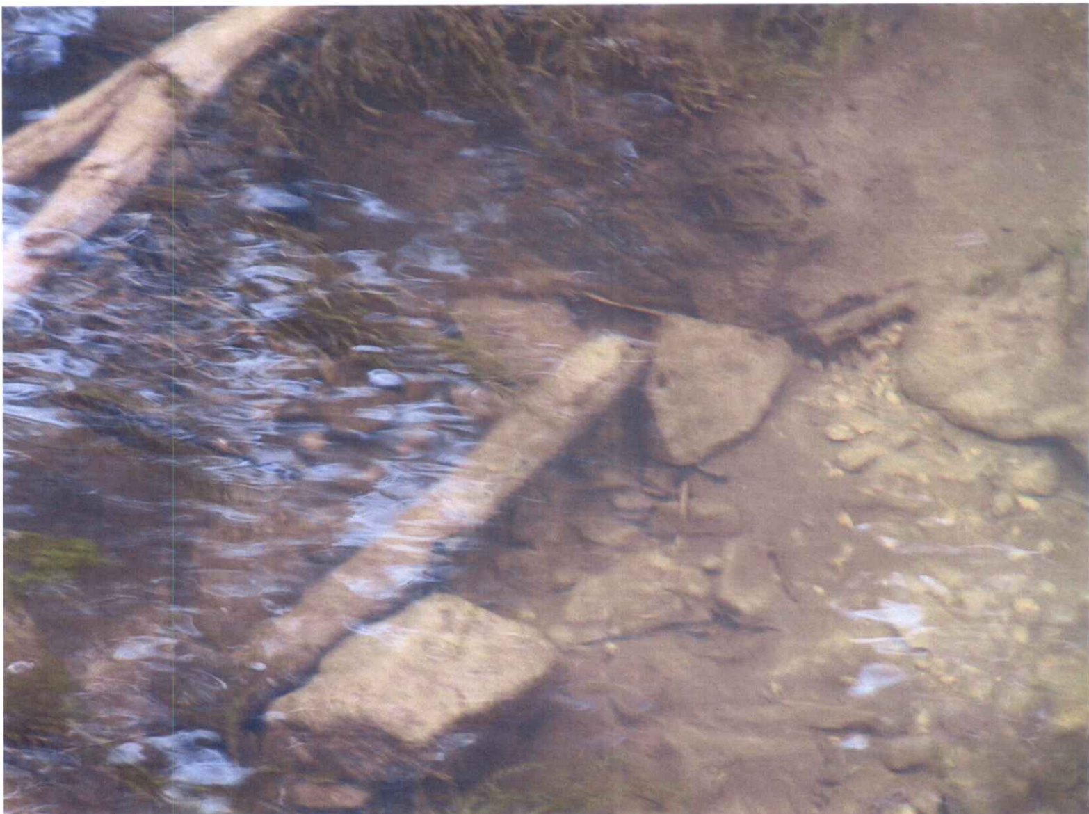
Inlet Pipe for Pump
