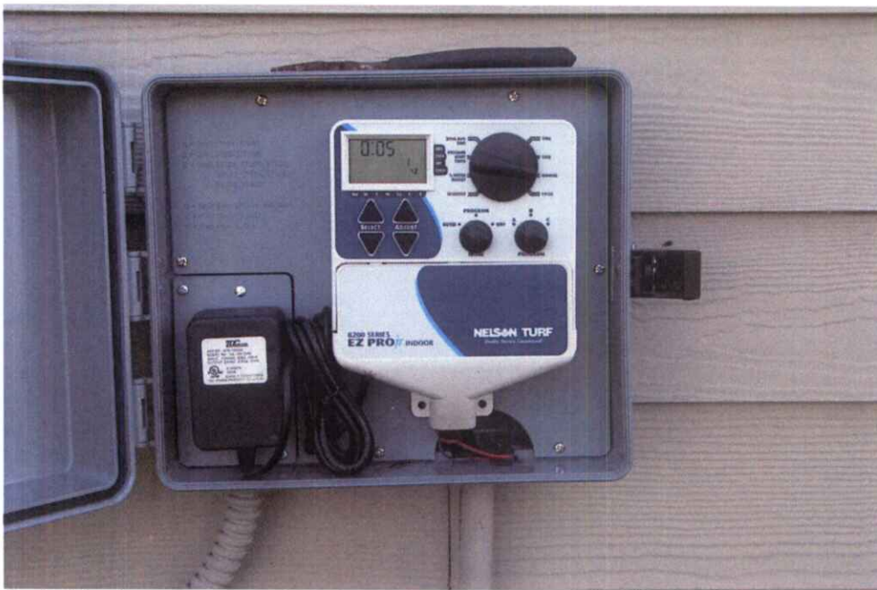
Sprinkler box that runs the system for the backyard and pasture
