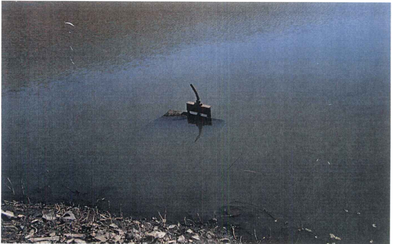
Photo #6: Gate frame sticking up in the reservoir.
