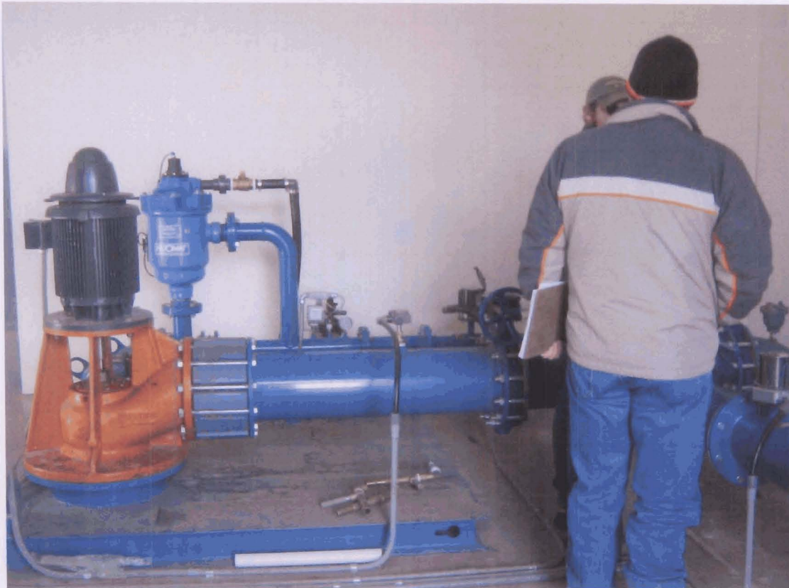
Recirculating and Irrigation Pumps and Water Meters
