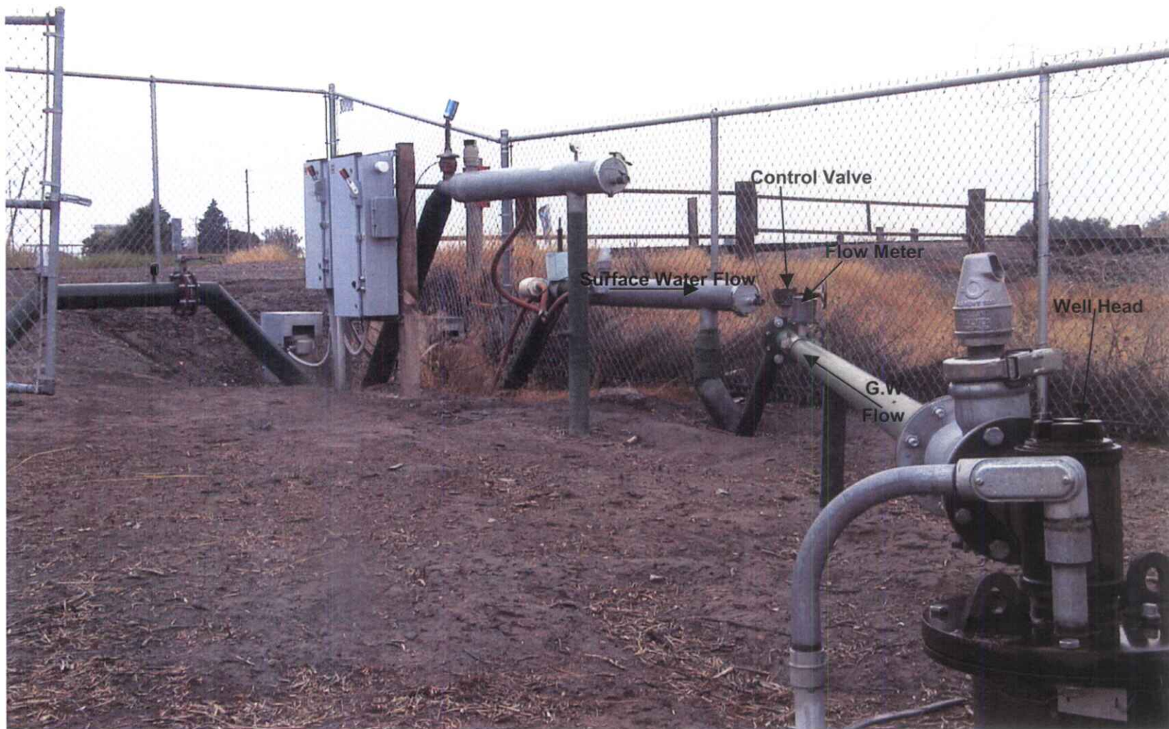
Point of diversion: Ground water well at right in foreground. Surface water pump system at right in background commingles water with water from well. Totalizing flow meter is positioned upstream of control valve that opens ground water flow into distribution line. Surface water pump system at left is a separate system.
