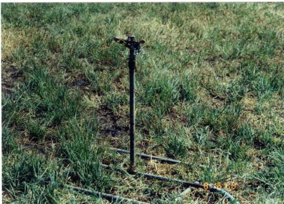
Photo 4. Showing typical Irrigation Sprinkler.
