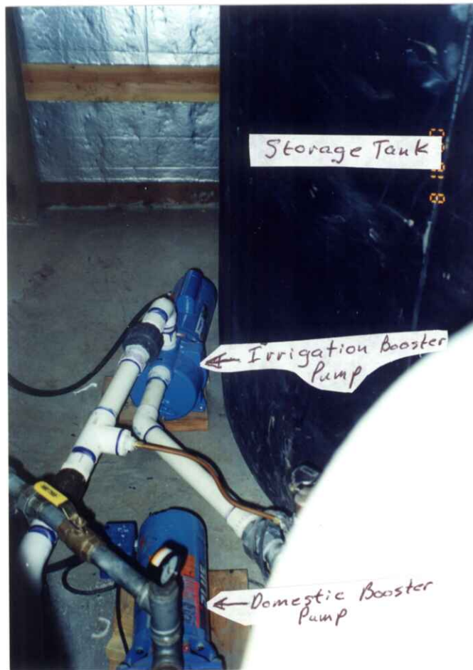
Photo 3. Inside of Well house.
