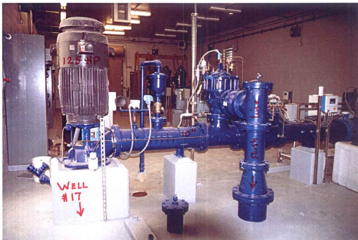
Figure 13. July 11, 2006 photographs inside of the Caldwell Well #17 pump/control house. Lower view looks west and shows the 125 HP Emerson drive motor and discharge-head on the Well #17. The upper photo is a closer look at the base of the discharge head and the monitoring port (measuring point) protruding from the concrete pump base of the well head. The electric well sounder in the foreground was used to measure water levels during the licensing examination.
