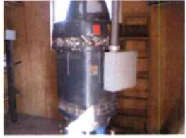
150 HP IRRIGATION PUMP
