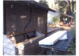
95-9273 Pump Shelter Insulated Cover.JPG
