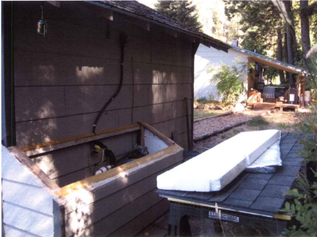
95-9273 Pump Shelter Insulated Cover.jpg
