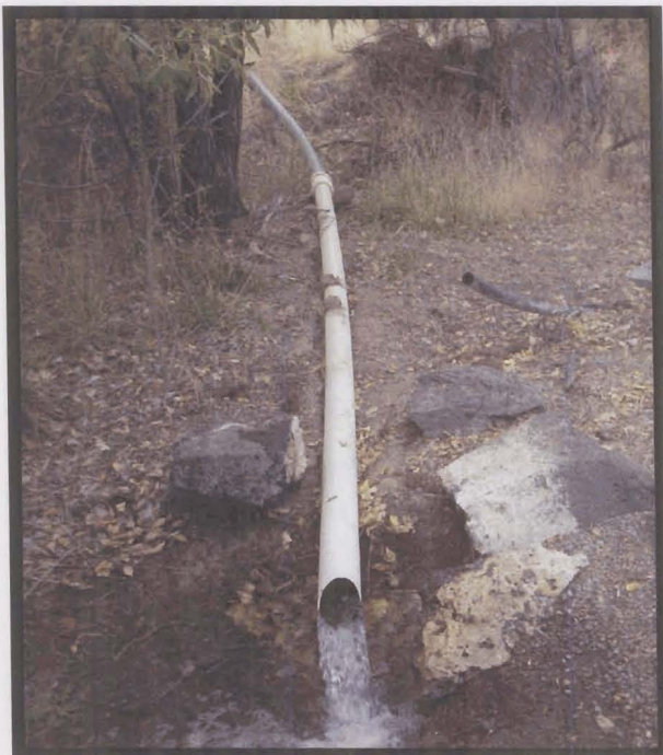
Discharge pipe where measurements were taken.
