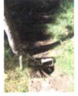
95-9252 Removed lid at Collect box.JPG
