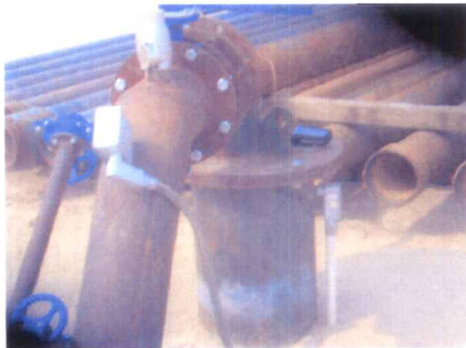
Well #2: 16-inch Casing, 200-hp Submersible Pump NWSE, Section 7 (also contains 7.5-hp submersible pump for permit 63-12569)
