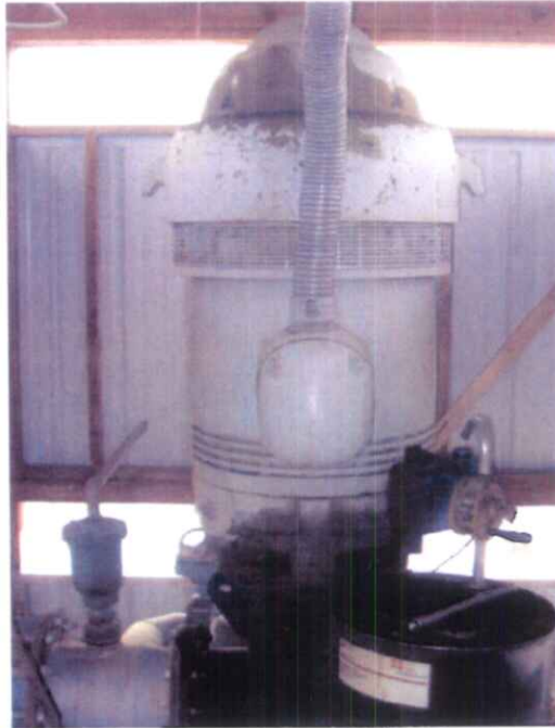
Well #1: 16-inch Casing , 300-hp Turbine Pump NWNW, Section 18 (Gov Lt 1)
