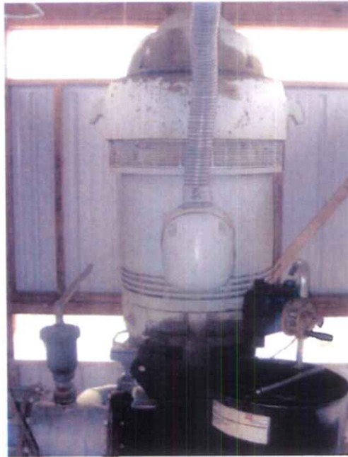
Well #1: 16-inch Casing, 300-hp Turbine Pump NWNW, Section 18, T6N, R3W (Gov Lt 1)
