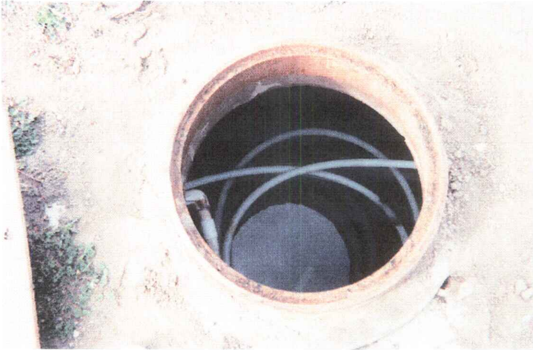
Hot water sump with discharge piping from patio & glycol heating systems.
