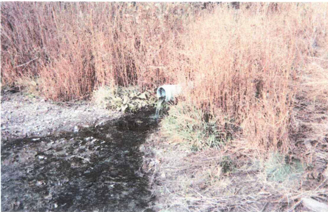
6" Dischage pipe to reservoir @ outfall location
