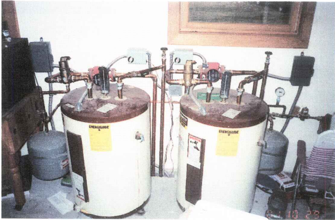
Glycol system hot tanks to boost glycol temperature to system.
