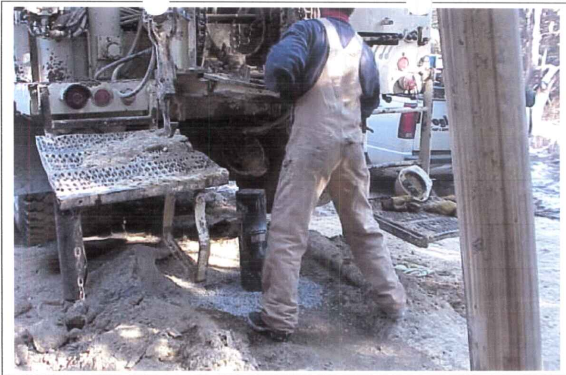
Photo 1: Well Casing, Drilling permit 789073 completed 11-1-02. WR Permit 87-10017. T43N, R05W, S15, NWSE.
