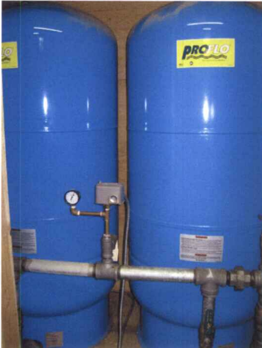
94-7394 Domestic Pressure Tanks in barn
