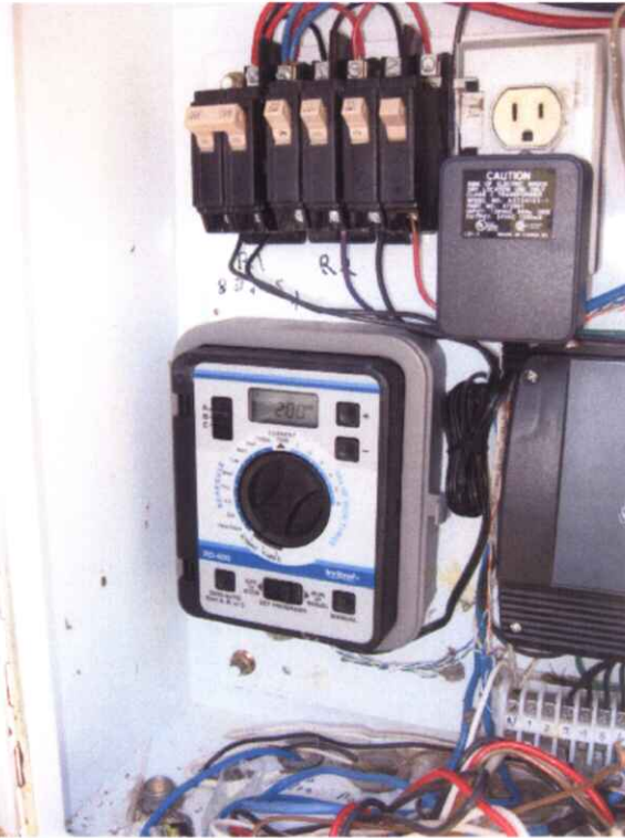
94-7394 Irrigation System Timer Controls
