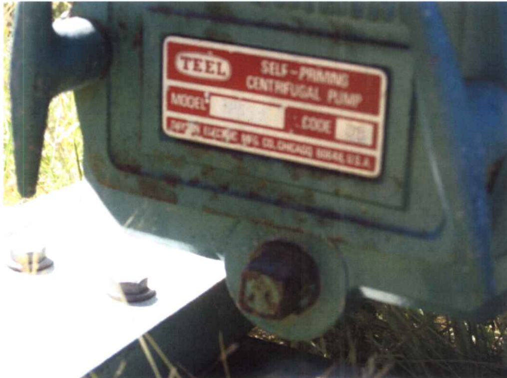
95-9060 Centrifugal pump on mobile dolly
