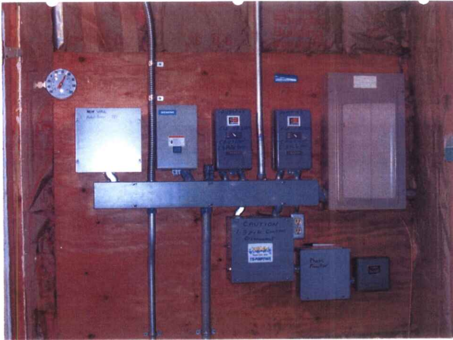
95-9251 Electrical Boxes in Pump House
