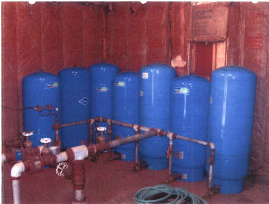
95-9251 Pressure Tanks in Pump House
