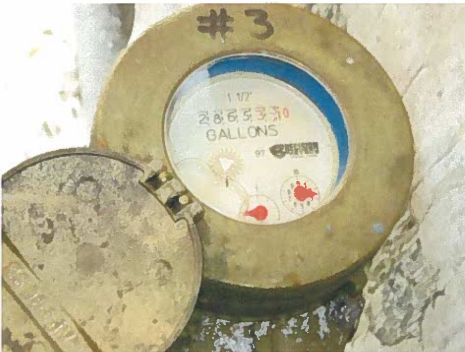
95-8834 Well 3 Analog Flow meter reading near start of Field Exam flow test
