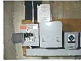
95-8834 Pump house electrical.JPG
