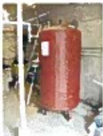
95-8834 Unused pressure tank in Pump House (Part...
