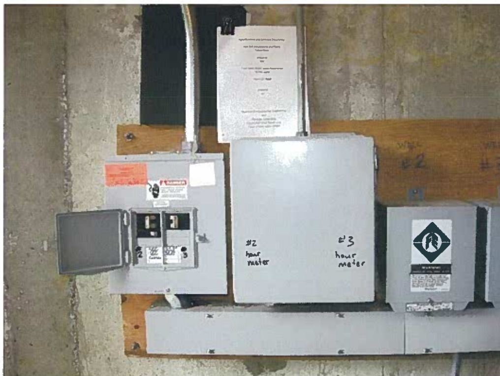
95-8834 Pump House Electrical
