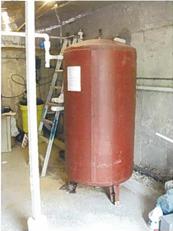
95-8834 Unused Pressure tank in Pump House (Part of 95-8517 System)
