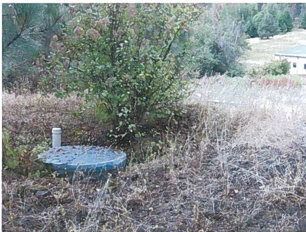
95-8834 Earth cover reservoirs next to pump house
