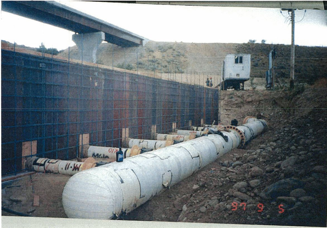
Discharge Manifold March, 1996:
