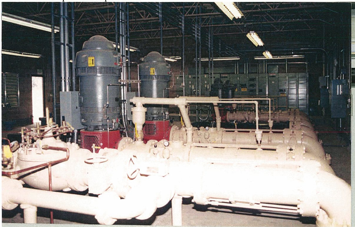
Interior of Pump House April 1998
