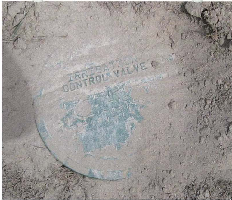
FIGURE 4: Irrigation control valve box
