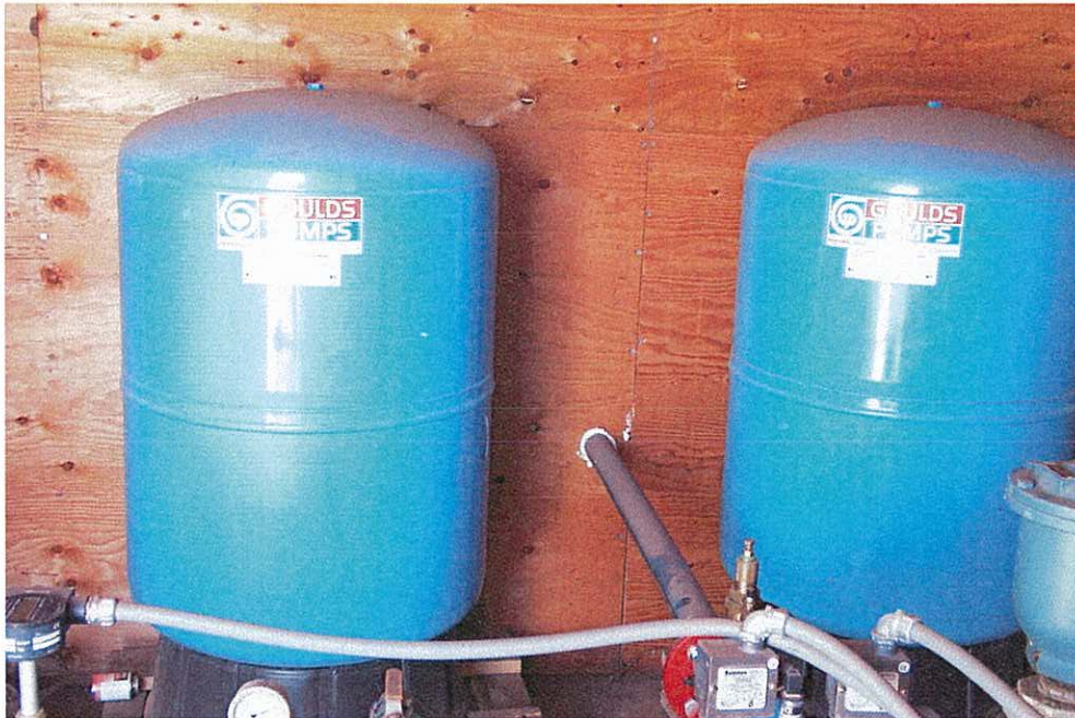
2x250 gallon holding tanks as part of well #2 diversion works
