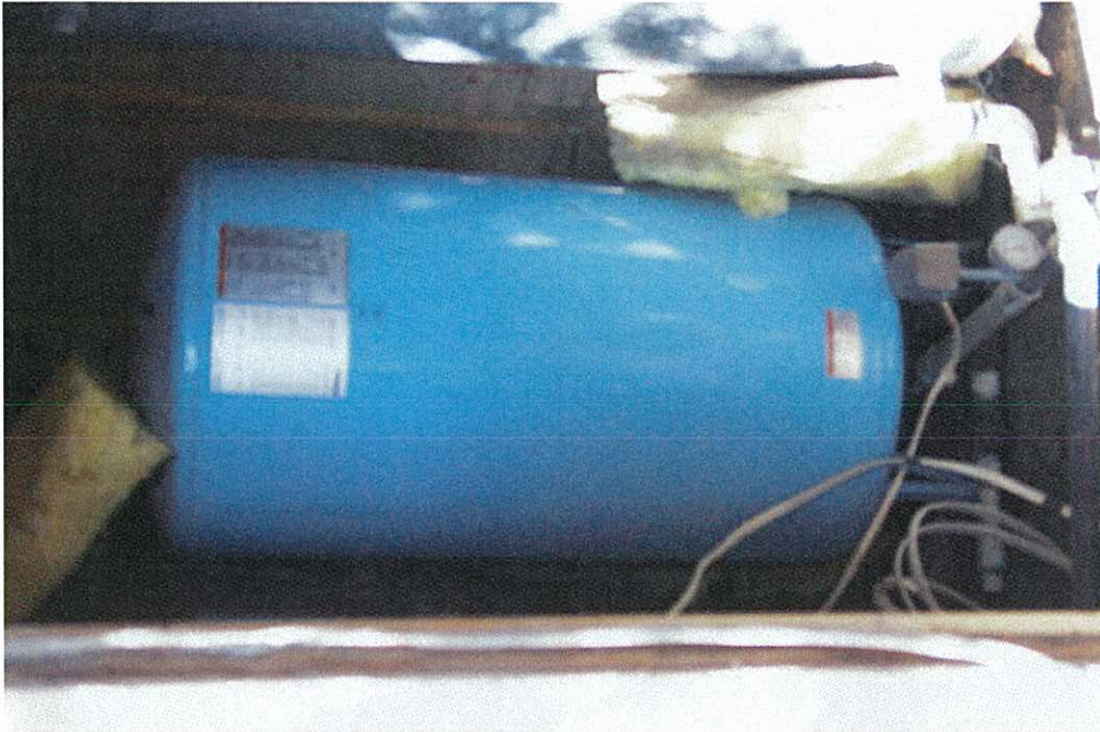
300 gallon holding tank for well #1
