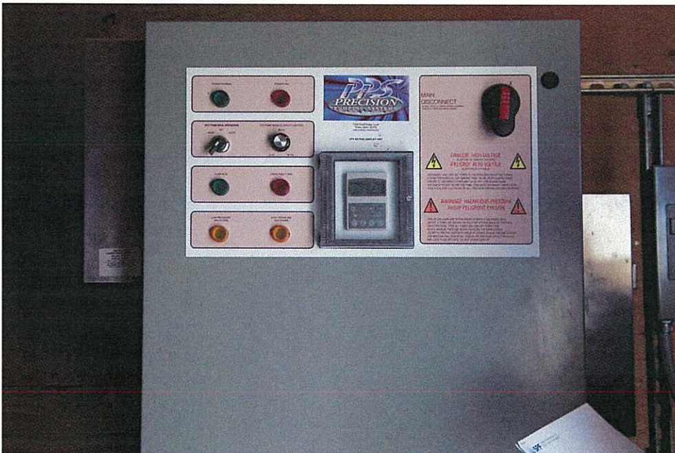
Control panel for well #2 located near the base of driveway
