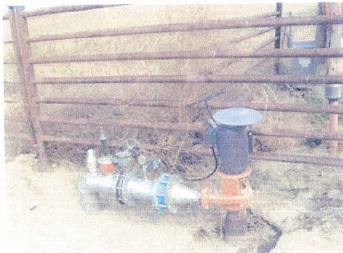
Booster #5: 7.5-hp NWNE, Section 7 Used for Kifco "Big Gun" Water Wheel Sprinkler
