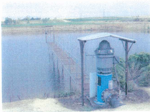
Booster #2: 75-hp SWSE, Section 7
