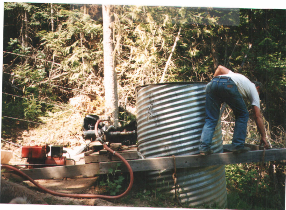
SPRING w/ ← Pump & generator
