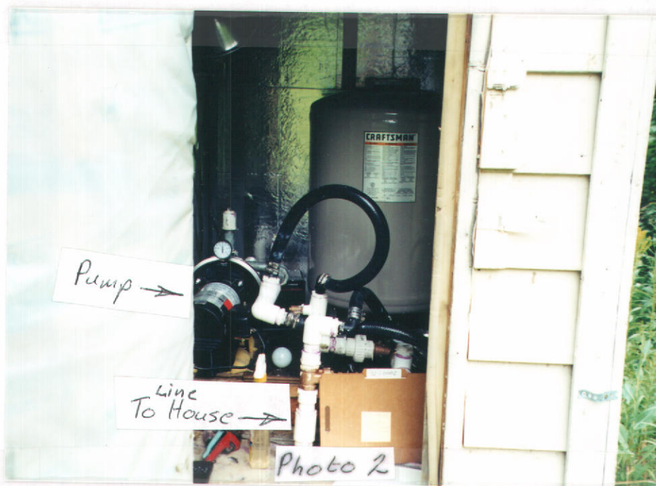
Photo 2. Showing Inside Pump House.
