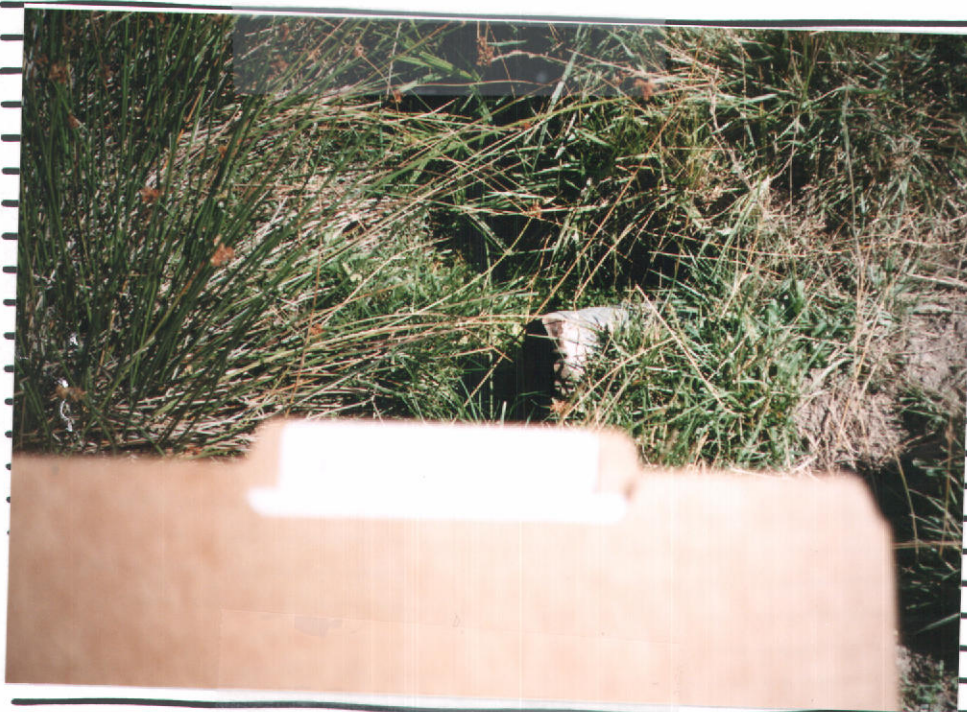
4" pipe draining into storage pond
