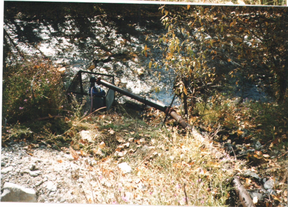
Point of Diversion & Pipeline
