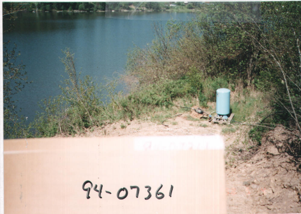
1/2 Hp Pump Pressure Tank
