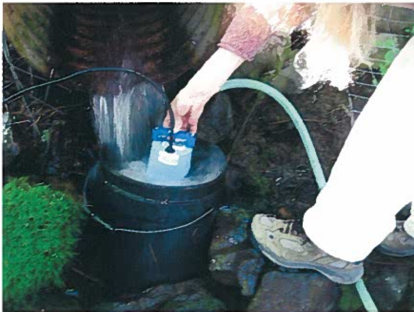
1/6 Horsepower Electric Submersible pump at POD
